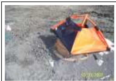
Inlet protection improperly installed
