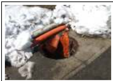
Inlet protection requiring replacement
