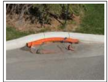
Street Inlet Protection
