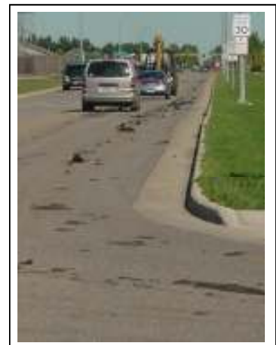
Sediment tracked onto roadway
