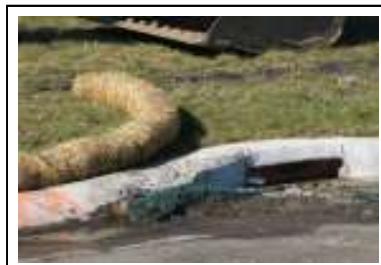
Damaged inlet protection
