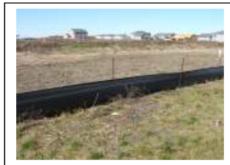
Standard silt fence
