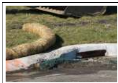
Damaged inlet protection
