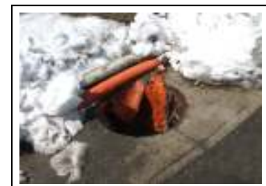
Inlet protection requiring replacement
