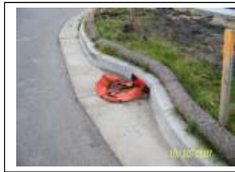
Street Inlet Protection
